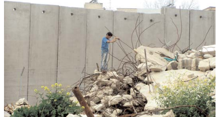
This home in Nazlat Issa has been destroyed to make space for the construction of the Apartheid Wall.
